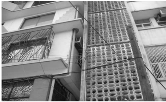
Figure 2 Two buildings without sufficient distance in between
