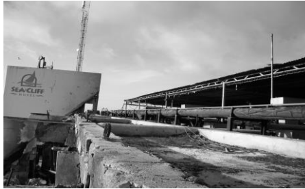
Figure 1 Fire gutted Sea Cliff Hotel in Dar es Salaam
