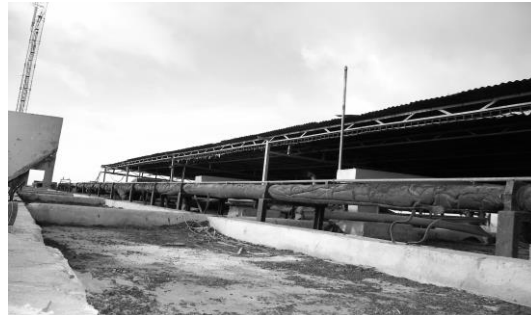
Figure 4 A duct which caused the spread of fire.
