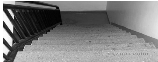
Figure 11 Stairs along the fire escape route as it is shown in Figure 12.
