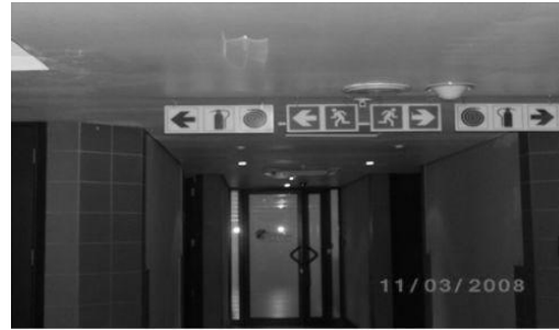
Figure 10 Fire proof doors.
