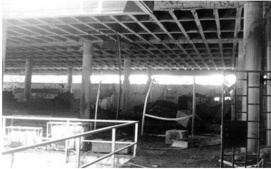
Figure 8 Fire gutted office partition walls at Ushirika building in Dar es Salaam.
