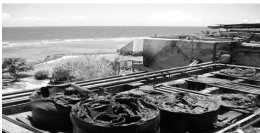
Figure 6 Fire gutted plastic water storage tanks
