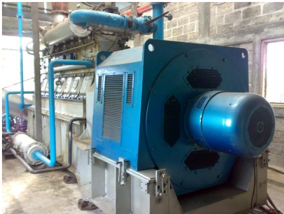
Figure 4. Gas engine power generation 400 kW
