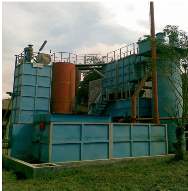
Figure 2. Fixed-bed updraft gasifier (Rice husk) PT. Natcham Wonosobo – Central Java
